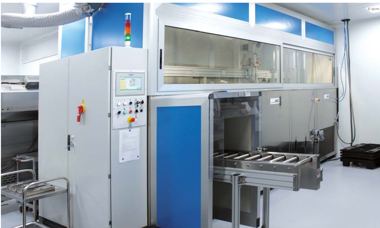
MEG's mixed-cycle cleaning plant.
