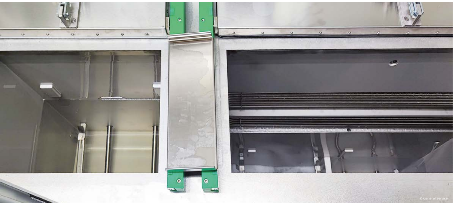
Two tanks of MEG's cleaning system.
