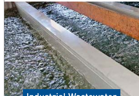
Industrial Wastewater Treatment
